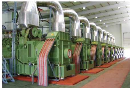
DRC - 33 MW Brazzaville powerplant
