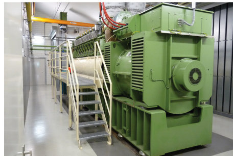
Netherlands - Kesteren 4.5 MW bio powerplant
